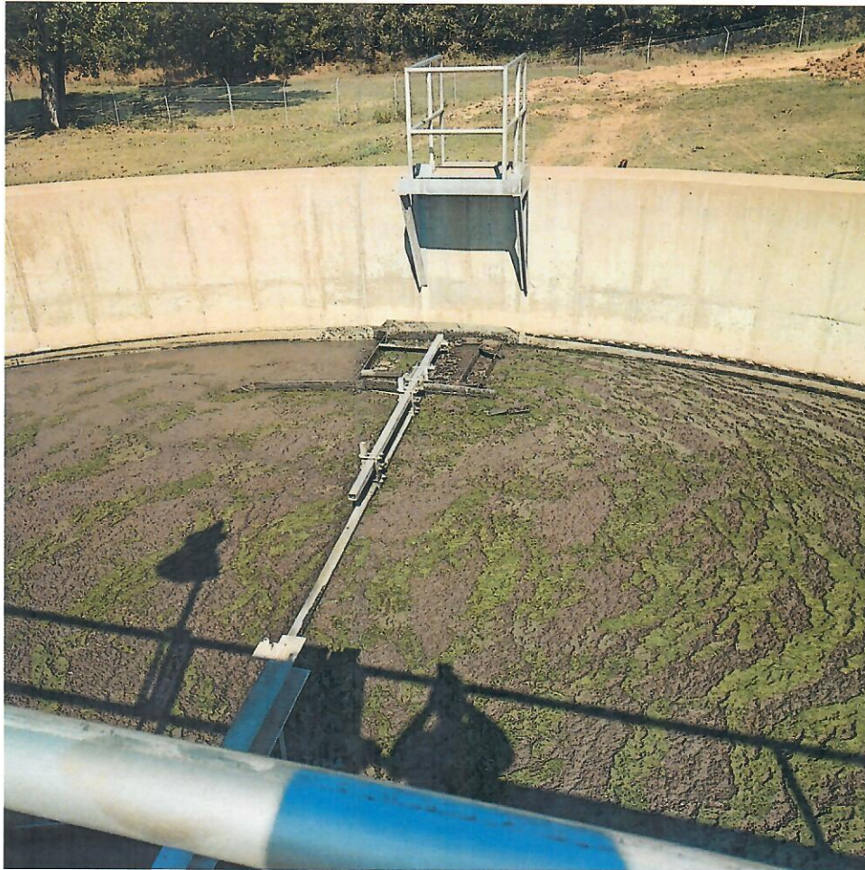
Clarifier Scum Arm Stuck
