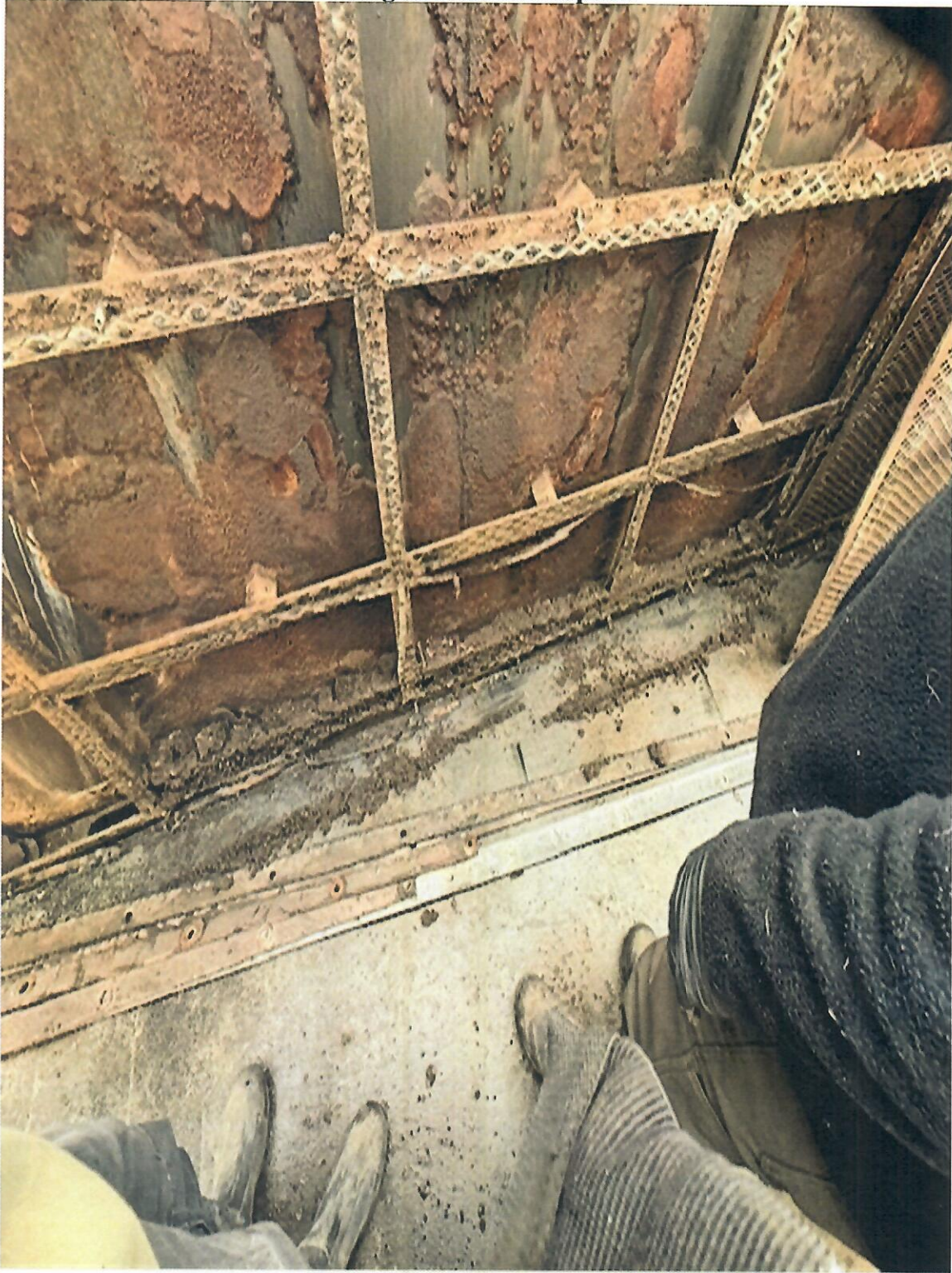
Sludge Box Before Repairs
