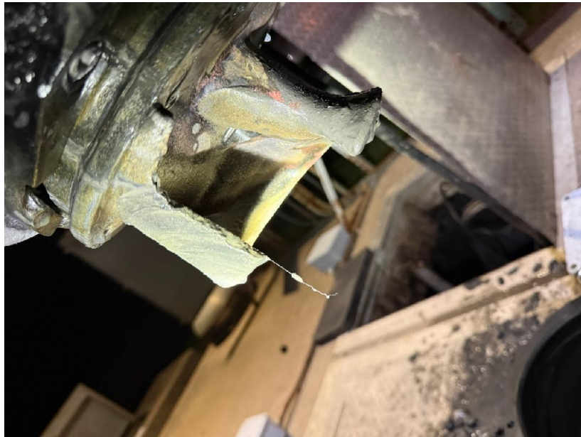
Impellor of the pump at Kimberly Clark Lift Station
