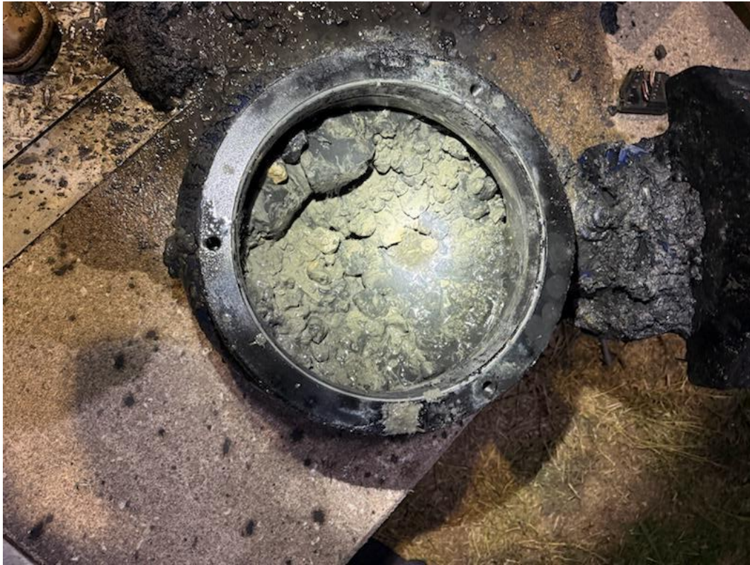
Rocks and debris inside the lift station pump
