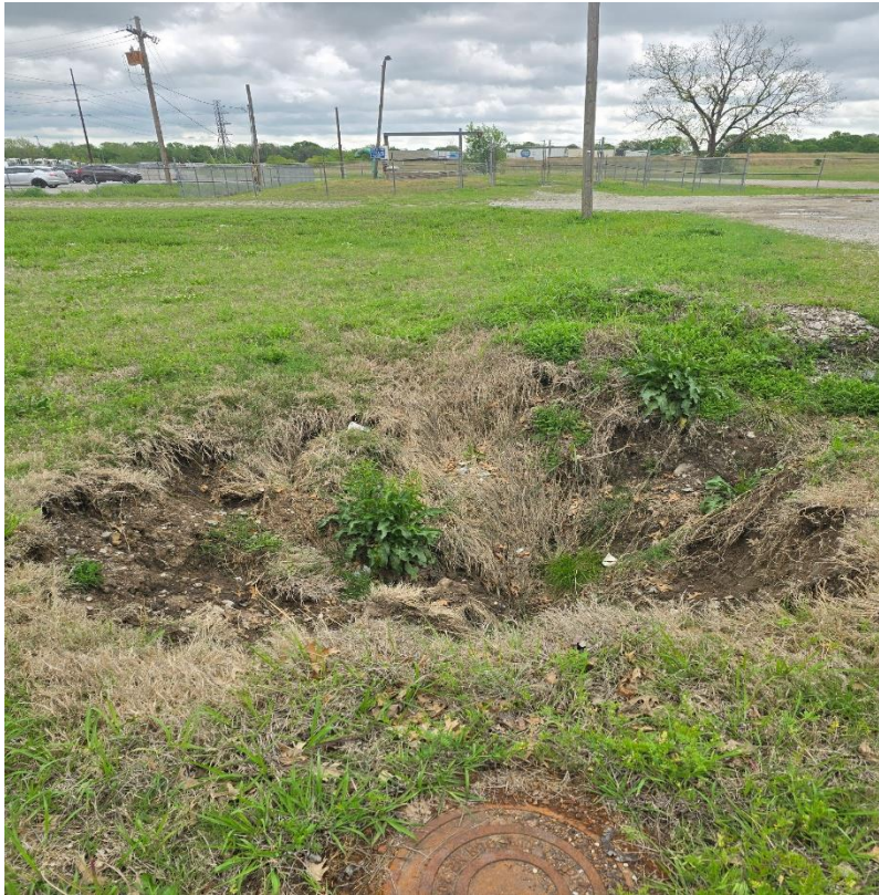
Kimberly Clark Lift Station sink hole
