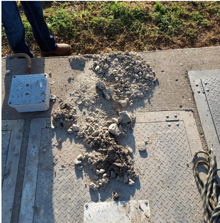
Debris Removed from the pump and debris in the lift station
