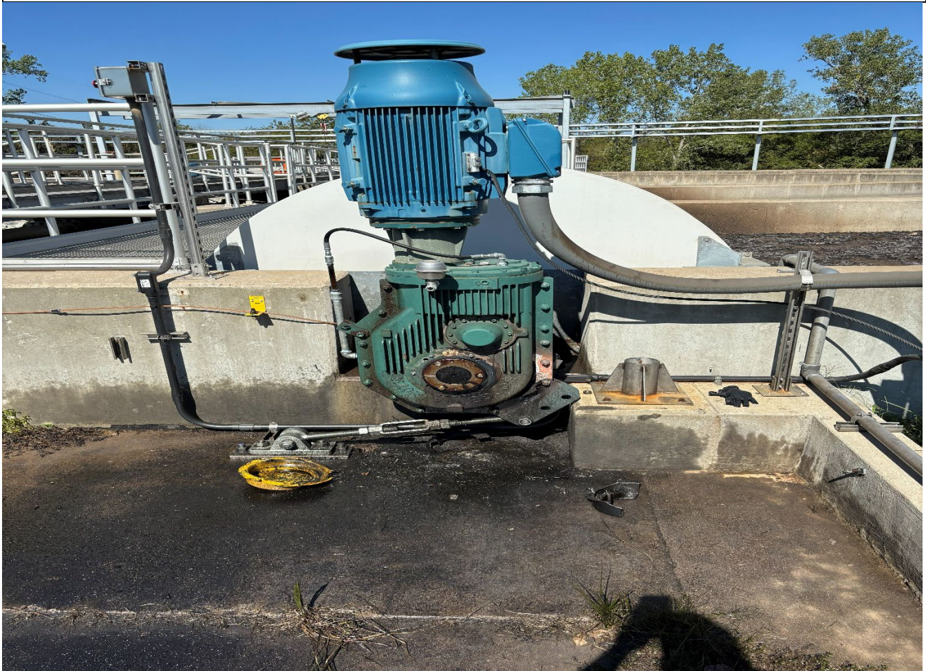
Damaged Gearbox for Aerator 2A
